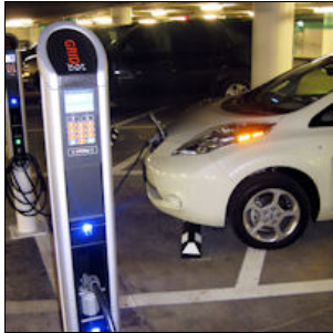
Electric Vehicle charging in Tranquillity Park Garage
